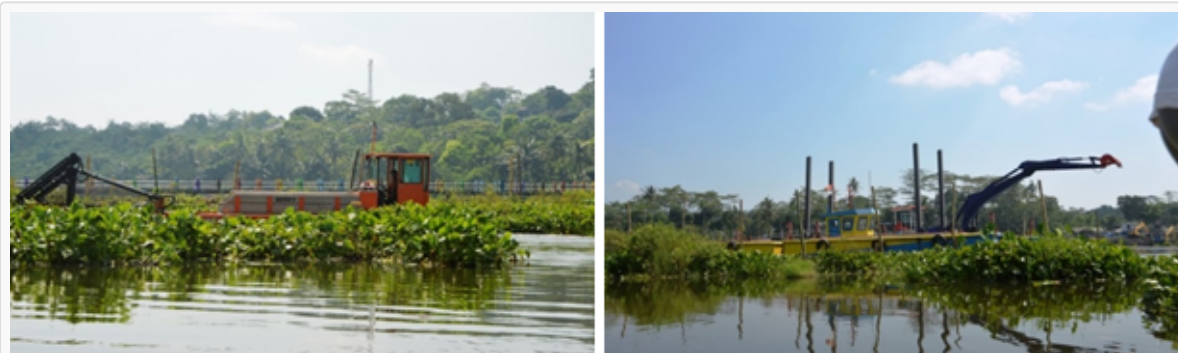
Figure 75. Two types of heavy equipment used to lift common water hyacinth in Rawapening
